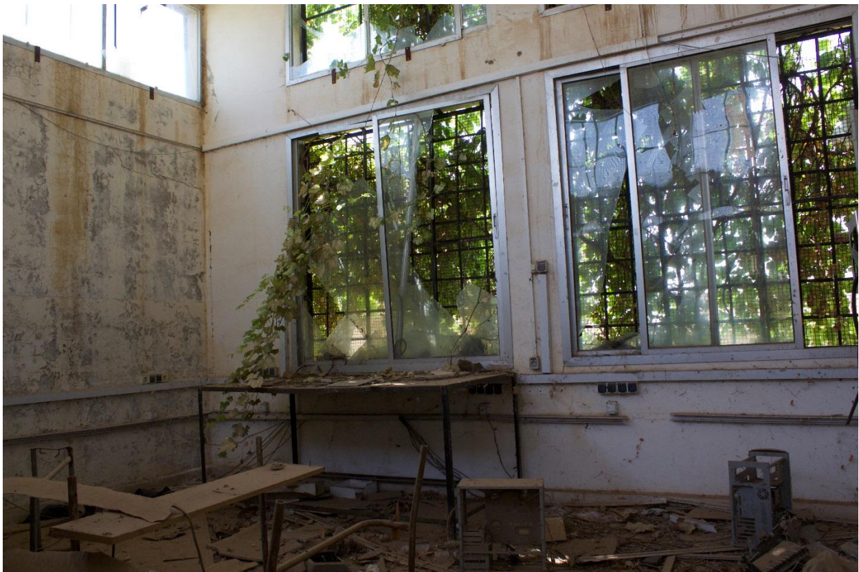
A school in North East Syria that has been occupied by several armed groups. War scars left behind include bullet holes, smashed windows, broken desks and sniper positions.
